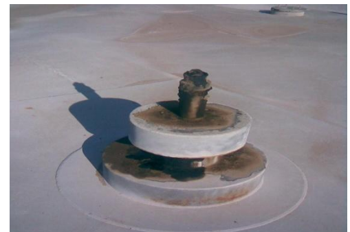
Figure 3- The vacuum breaker of tank
